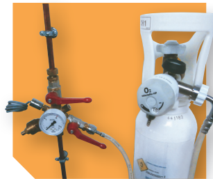
Supplying the network with backup cylinder
